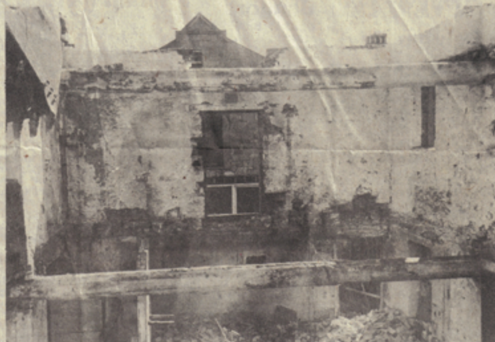
Demolition work on the old warehouse, where the beams made out of ship's timbers can be seen.
